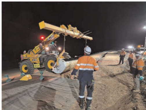
Figure 2. Innovative High Friction Angle (HFA) BGMs being deployed on slopes for mine waste capping and environmental protection. Northern Territory, Australia.
