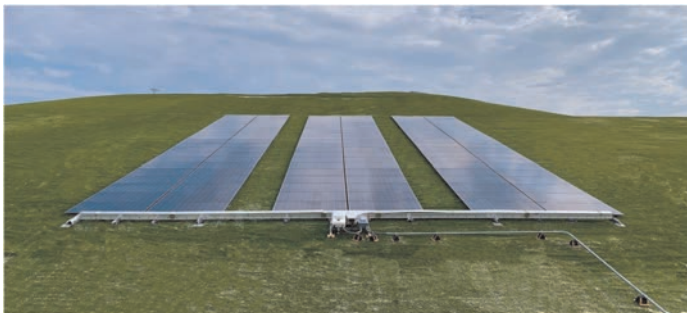
Figure 7. PowerCap installed on engineered turf cover at a confidential CCR impoundment, Southeastern US.
