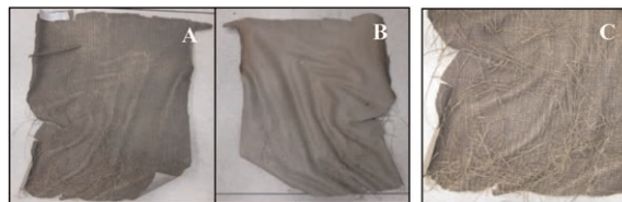
Figure 4. PVC-P geomembrane sample extracted from the north slope crest 258 months after re-waterproofing. A: external face, in contact with the HDPE geomembrane, B: internal face, in contact with the geotextile, C: detail of the state of the external face of the geomembrane.
