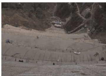
Figure 10. Berm provided to collect & drain surface water.
