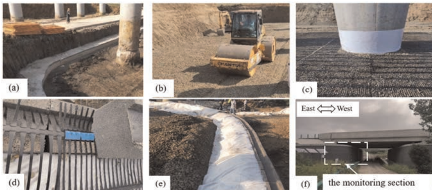
Figure 1. Construction of the MSE wall: (a) Strip footing; (b) Large-sized roller compactor; (c) Geogrid bypass the pile; (d) Connection between geogrid and blocks; (e) Filtration drainage layer; (f) Photo of the bridge supported by the MSE wall with embedded piles after the completion of the construction.
