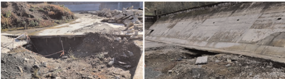
Figure 5. Pictures of the 2020 failure.
