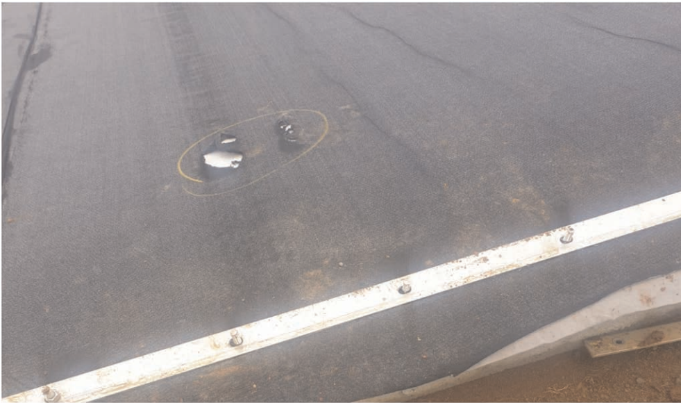
Figure 5. Holes in a conductive composite made by workers walking on it. These required patching to ensure adequate conductivity.
