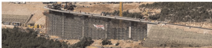
Figure 5. Replacement of external portions of the Brijesta viaduct with reinforced earth embankments (total length about 200 m, maximum height about 15 m).
