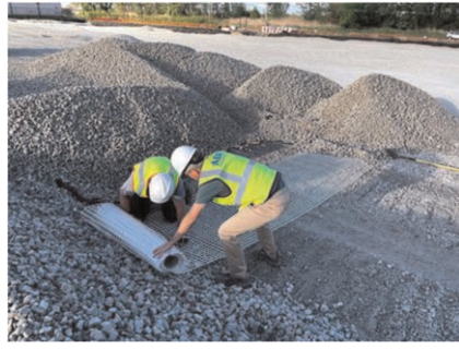
Figure 6. Photograph of PHL Ron installation.
