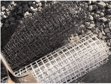
Figure 5. Photo of GS installed at PHL Ron.
