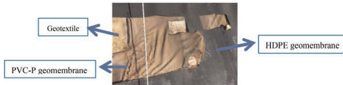
Figure 3. Appearance of the PVC-P geomembrane under the HDPE geomembrane in the crest area of the north slope at 216 months.
