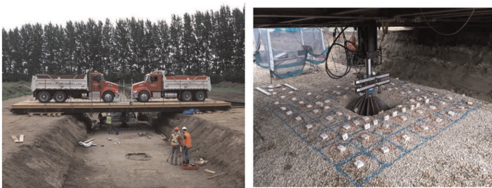
Figure 1. Saskatchewan University full scale temporary working platforms testing (Left: general set up, right: platform after the test).
