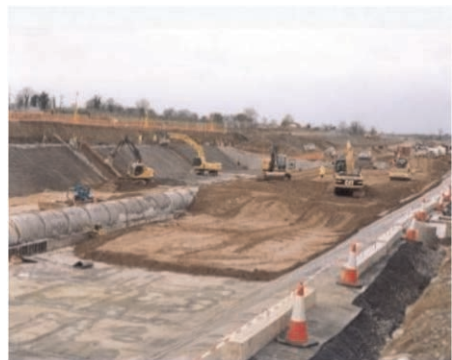
Figure 8b. Membrane over central collector.
