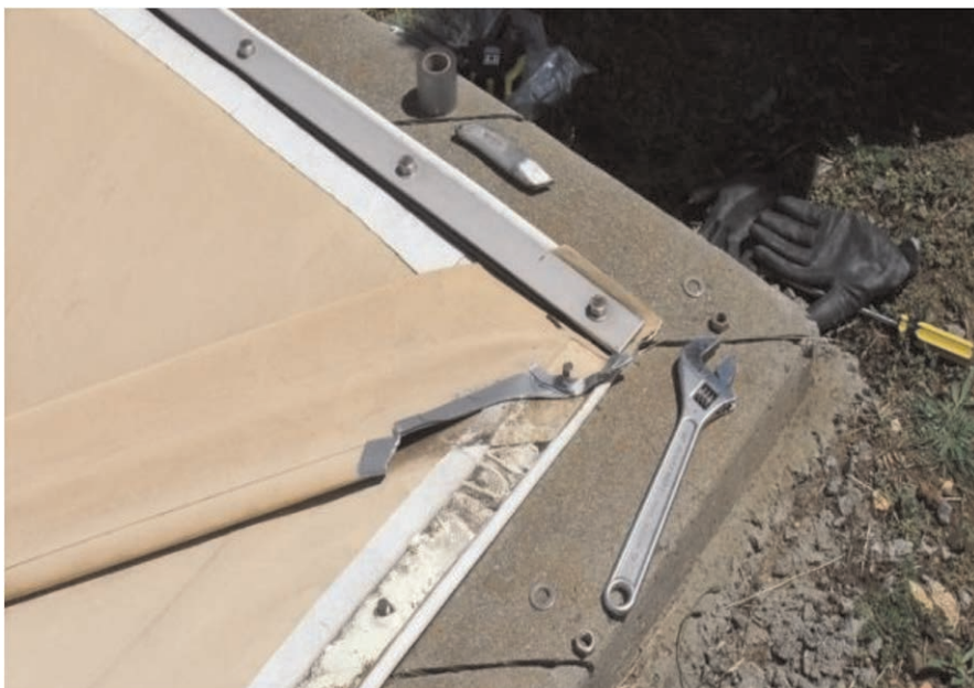
Figure 1. A small cover material sample taken from a ballast tube partly under a batten bar.
