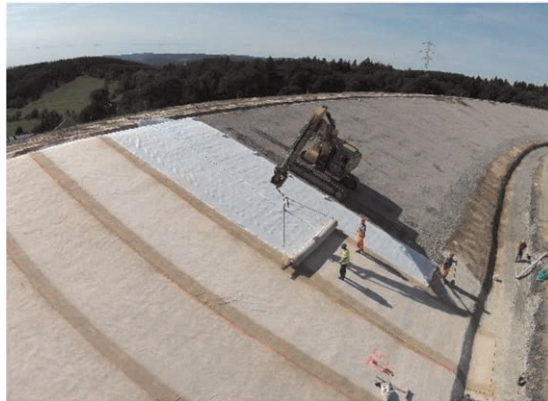
Figure 17. Geosynthetic drainage composite mat (white color) with a Geosynthetic Clay Liner (GCL, light brown) on top as sealing system.
