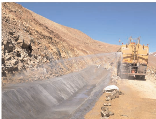
Figure 2. GCCM hydrated by surface spraying resulting in pooling water in the invert. These parts of the GCCM structure cure in immersed conditions.
