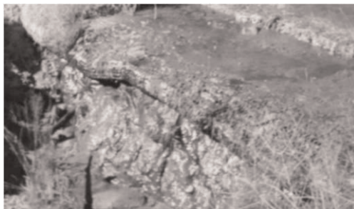
Figure 25. Clogging of a geotextile filter caused by ochre formation.
