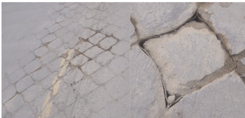
Figure 6. Fail presented in a soft soil with high fines and water presence.
