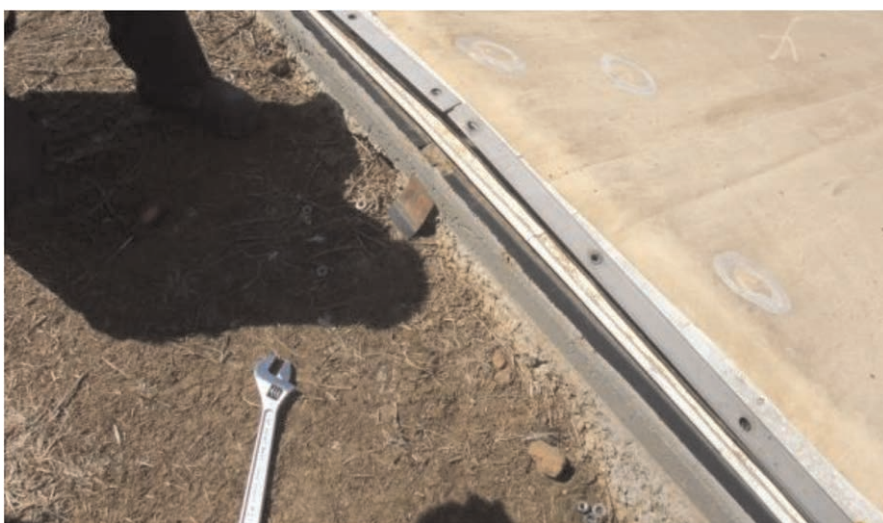
Figure 2. A small liner material sample taken from under a batten bar. This floating cover had many small marked holes which had been caused by embers from a grass fire.
