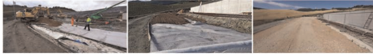
Figure 5. Construction phases of internal roads with the use of base geocomposite reinforcement.
