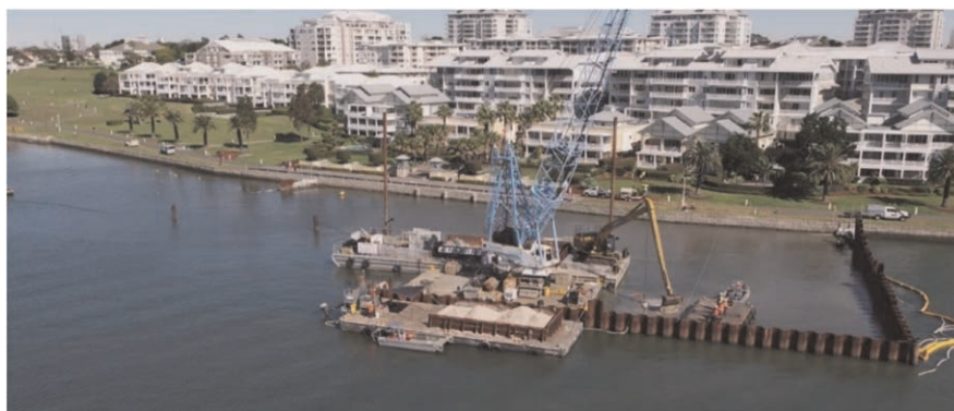
Figure 3. Site remediation in front of modern housing estate (Courtesy of HUESKER Australia).
