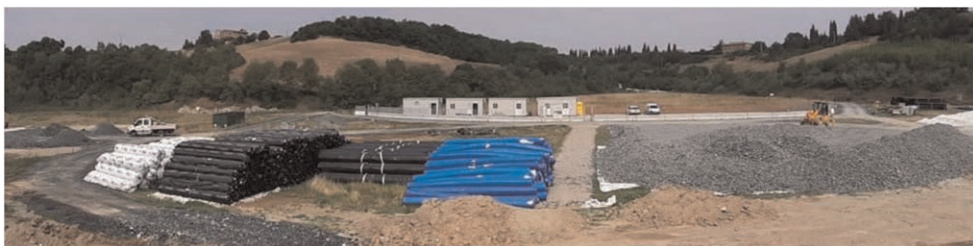
Figure 2. GCL and drainage geocomposite rolls stored on flat surfaces to avoid detrimental deformations.
