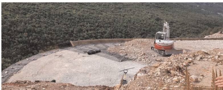
Figure 3. Construction phase of reinforced earth structure with mono-oriented extruded geogrids in HDPE.
