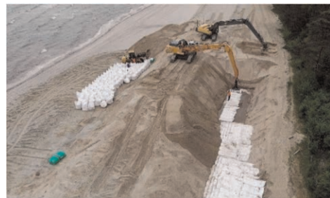
Figure 14. Installation of Geotextile Sand Containers as coastal protection measure in the dune core of the sandy beach, Lubmin Germany.
