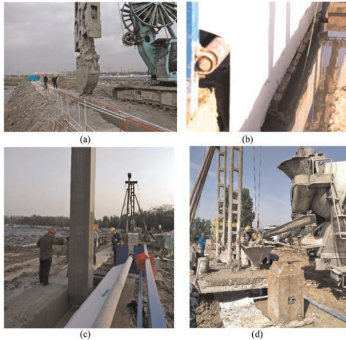
Figure 5. Construction of GCL composite vertical anti-seepage barrier: (a) Trench excavation, (b) Laying of GCL composite component, (c) Dropping down the joint box, (d) Pouring wall materials.
