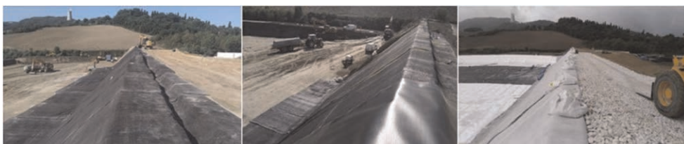
Figure 3. Slopes covered, from left to right, with the rough GCL, the HDPE liner, drainage geocomposite (slopes) and nonwoven geotextile (bottom).
