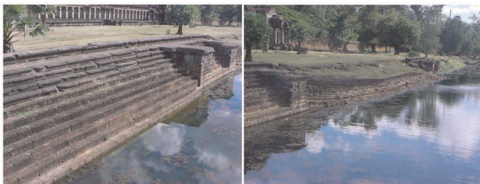
Figure 2. Adjacent portions of the steps showed a different behavior due to different boundary conditions. Left: dry assemblage of the steps; Right: Joint sealing (gray cementitious mortar) preventing drainage.
