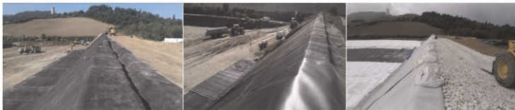
Figure 6. Slopes covered, from left to right, with the rough GCL, the HDP liner, drainage geocomposite (slopes) and nonwoven geotextile (bottom).
