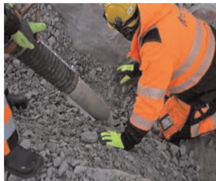
Figure 10. Removal of last part of granular material using a vacuum and by hand.
