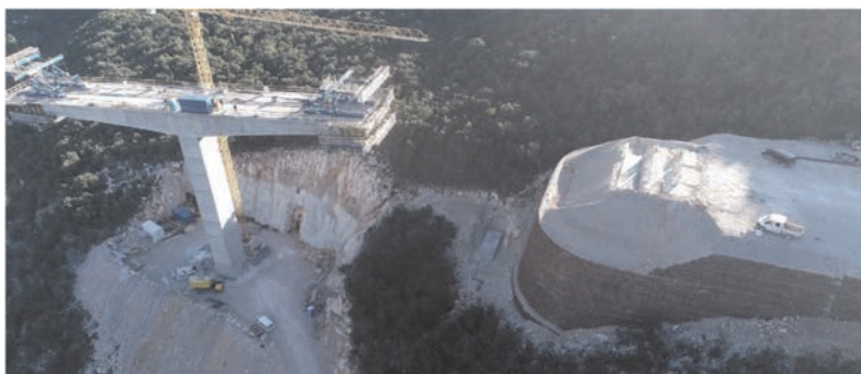
Figure 7. Aerial drone view of the U4 wing wall and abutment of the Dumanja Jaruga viaduct made with the reinforced soil technique with mono-oriented extruded geogrids in HDPE.
