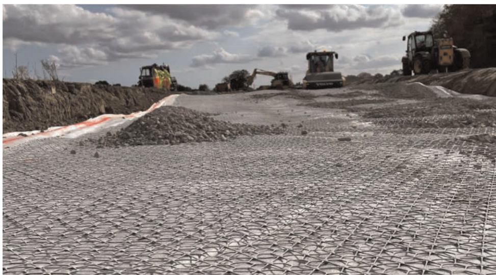
Figure 9. Installation of the pavement capping layer at North Heybridge (Tensar International Ltd).
