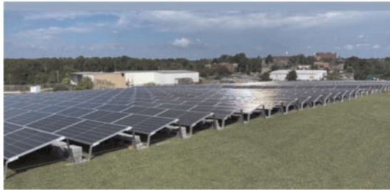
Figure 6. Community Solar farm installed on engineered turf cover at the Cranston Sanitary landfill, Cranston, RI.
