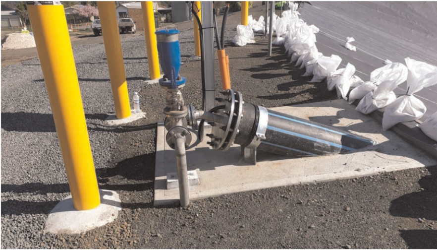
Figure 4. An underdrain water extraction system with a down the slope pipe with a bore pump.
