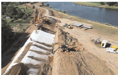
Figure 11. Installation Geosynthetic Clay Liner (GCL) on a levee reinforcement to replace a 1 meter thick clay layer (Beesel Netherlands).
