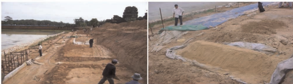
Figure 4. Overview of the working site and detail of the filling of the slurry trench.
