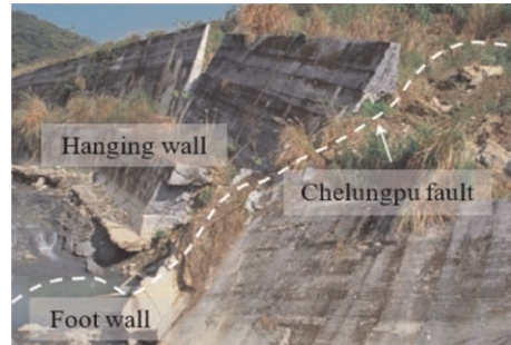
Figure 2. Failure of reinforced concrete revetments caused by Chelungpu fault (Chiang et al. 2022).
