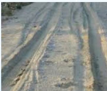
Traffic load-induced failure and rutting
