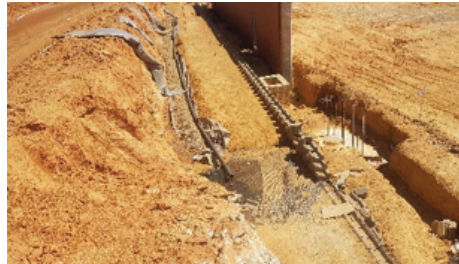
Subsoil drain and band drain at the back of a GSY wall
