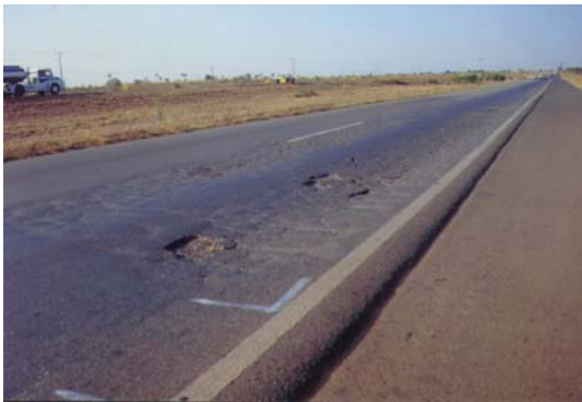
Damages in a conventional pavement
