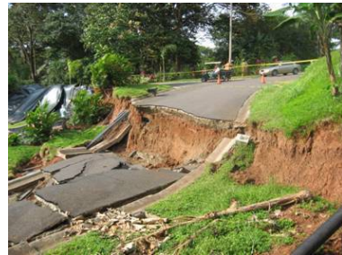
Figure 1. Initial state: Failure of the existing soil and road
