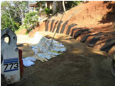
Figure 4. Installation of sacks (filled to a 1/3 of their volume with organic soil) in the façade
