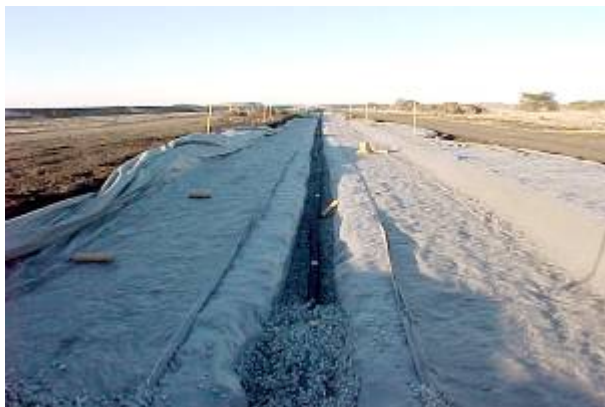
Figure 59: Tailings dam perimeter drain
