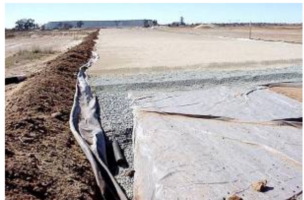
Figure 60: Tailings dam perimeter drain
