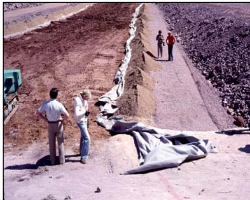
Picture - 7 Close up of filter system at Mokol Dam (Photograph kindly supplied by Jean-Pierre Giroud)
