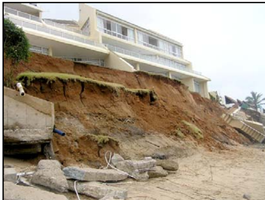
Picture 17 - Damage from rough seas
