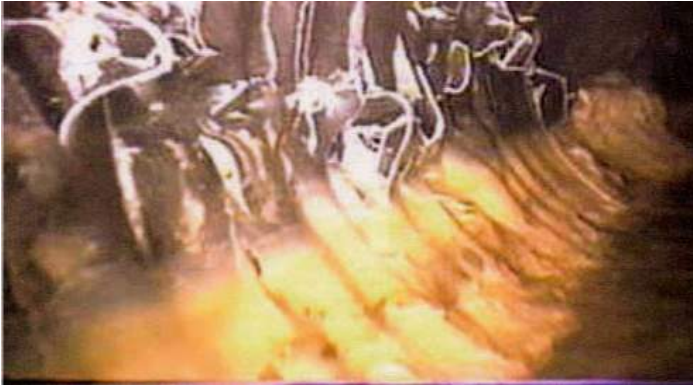
Figure 26. 0.6m diameter CPe Pipe wall buckling under 60m of ore (~ 1.0MPa)
