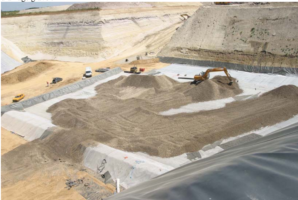
Figure 33. GCL used as a protection of the geomembrane at the Attainville MSW landfill (from Didier et al. 2006)
