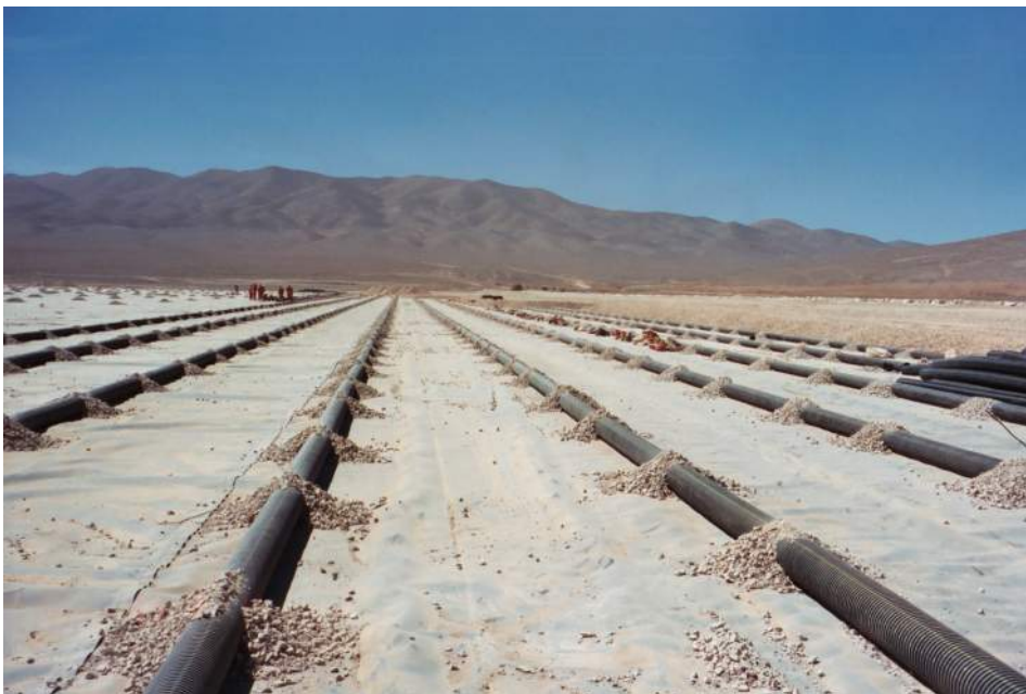
Figure 10. HLP corrugated polyethylene solution collection pipes
