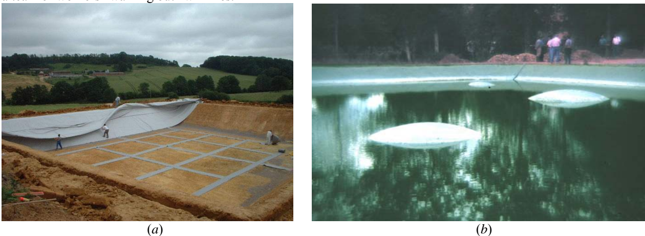
Figure 15. (a) Drainage strips at the bottom of a pond before lining; and (b) uplifted areas in a geomembrane
