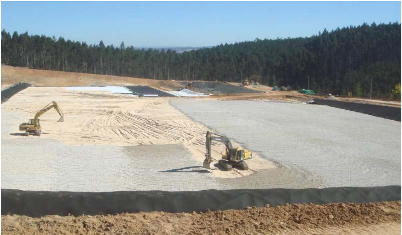
Figure 5. Placement of a drainage layer in a bottom landfill liner containing 0.2m of sand and 0.3m of gravel
