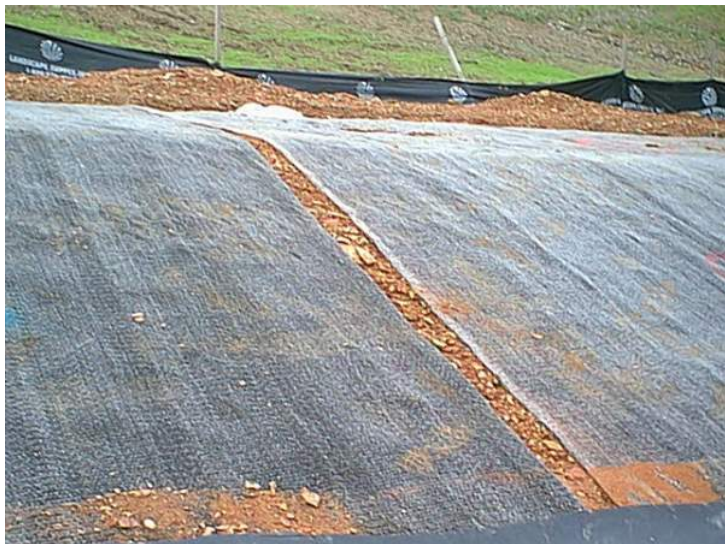
Figure 53. Photograph showing gap in GCL panels after removal of geomembrane (from Thiel & Richardson 2005)
