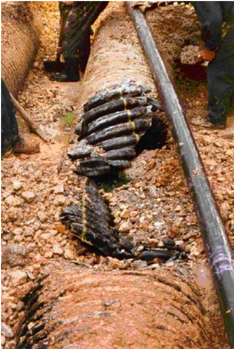
Figure 19. Pipe failure by crushing
