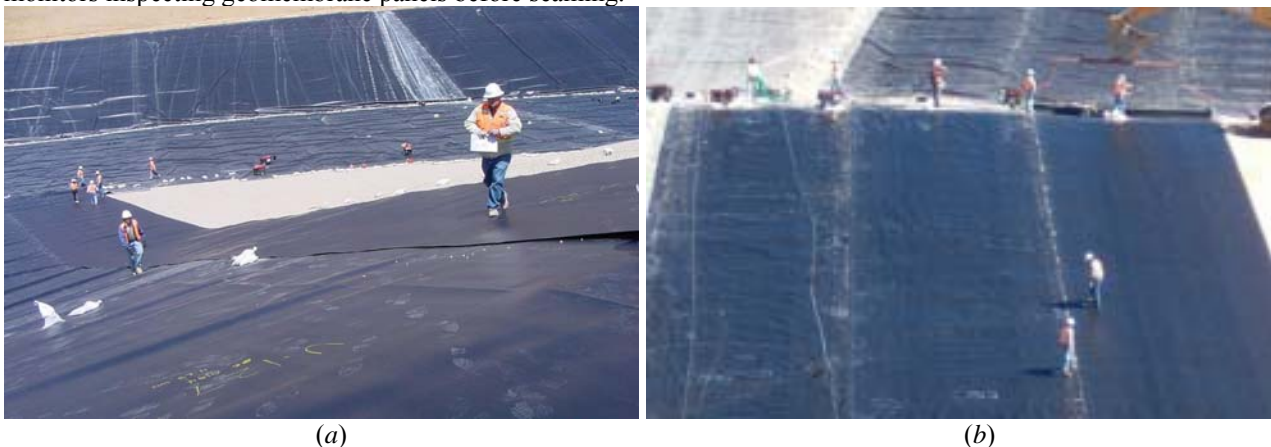
Figure 42. (a) CQA Inspection of Geomembrane Panel; and (b) Inspection of Several Panels Prior to Seaming (note panel and seam orientation)
