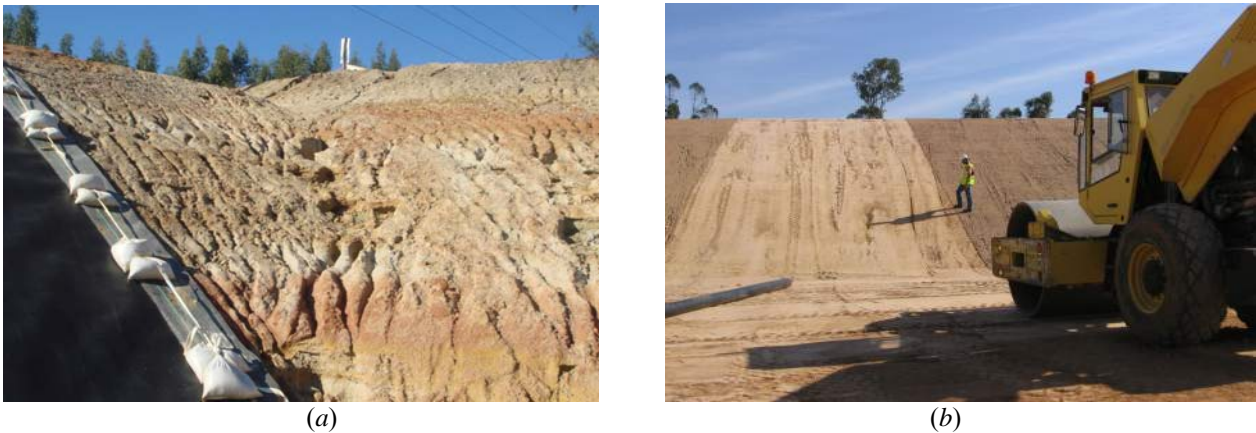
Figure 41. Illustrations of (a) poor subgrade quality and (b) good subgrade under construction
