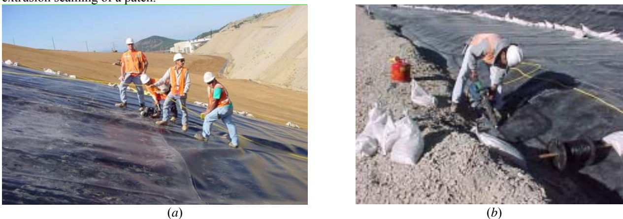
Figure 44. (a) Hot wedge seaming and inspection; and (b) extrusion seaming of a patch
