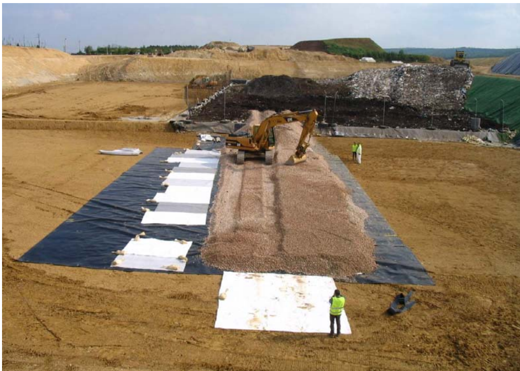
Figure 36. View of crushed gravel installation on testing pads (from Budka et al. 2007, reproduced with the permission from SITA France)
