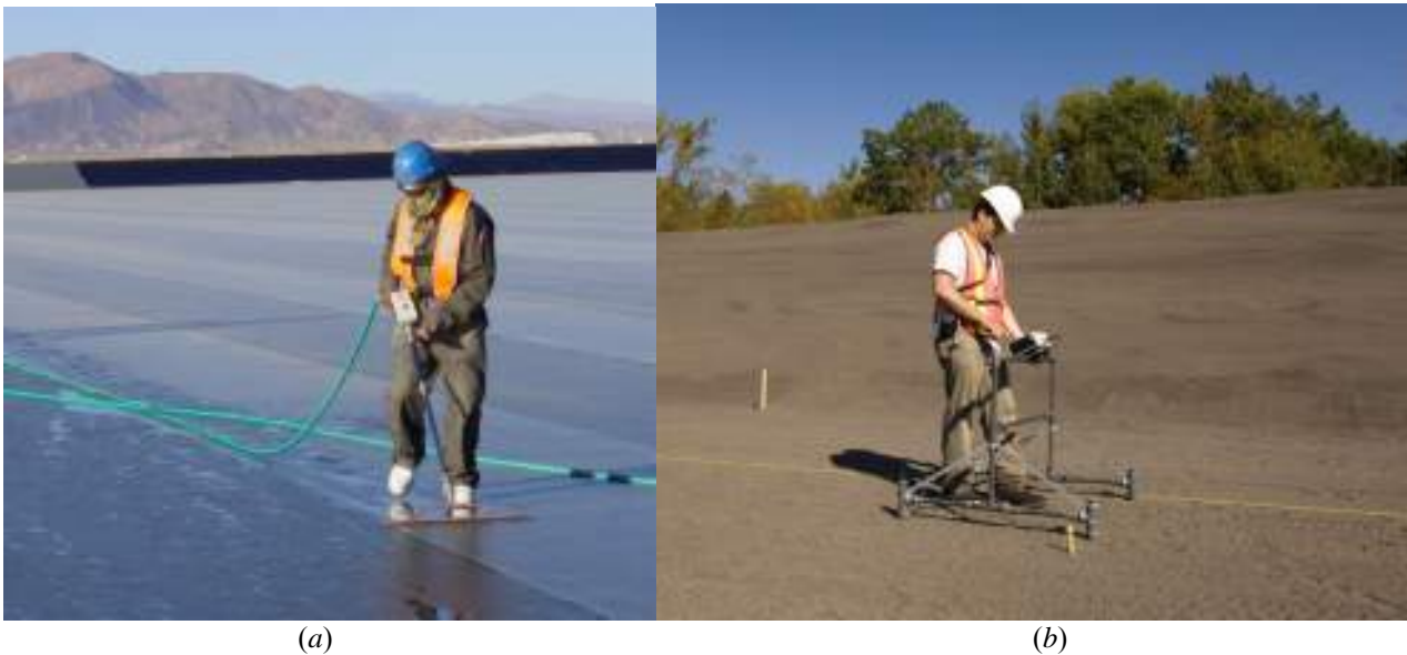
Figure 46. Electrical leak location survey (a) on exposed geomembrane; and (b) on covered geomembrane (courtesy of Solmers).
