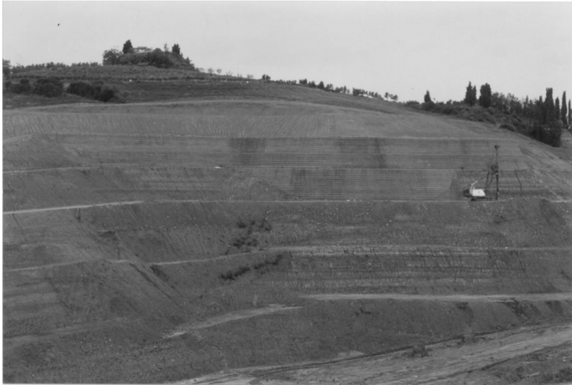
Figure 6. View of the northern slope with the reinforced earth walls. The "kelly" excavator is working at the intermediate diaphragm.
