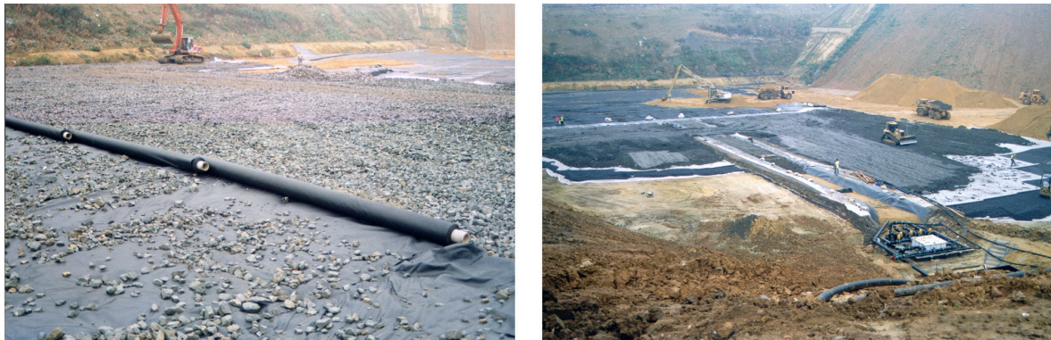
Fig. 1 and 2. General view of the basal layers with Terralys geotextiles being installed.
