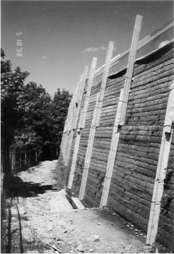
Figure 4: Safety railing and inclination guides
