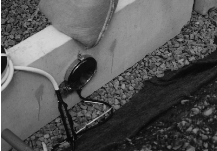
Photo-3 Earth pressure gauge (horizontal directions)
