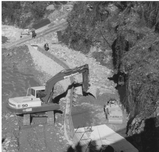
Figure 7. Construction of first layers of reinforced earthfill. In foreground the reinforcing metal braces.
