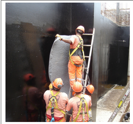
Figure 3: The installing of drainage's geocomposite for the first 4.50 m of height. in the wall.
