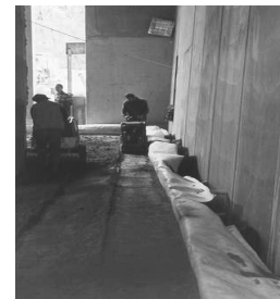
Fig. 4: Soil compaction in front
