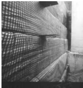
Fig. 12: Gap between the concrete facing and the geogrid reinforced wall
