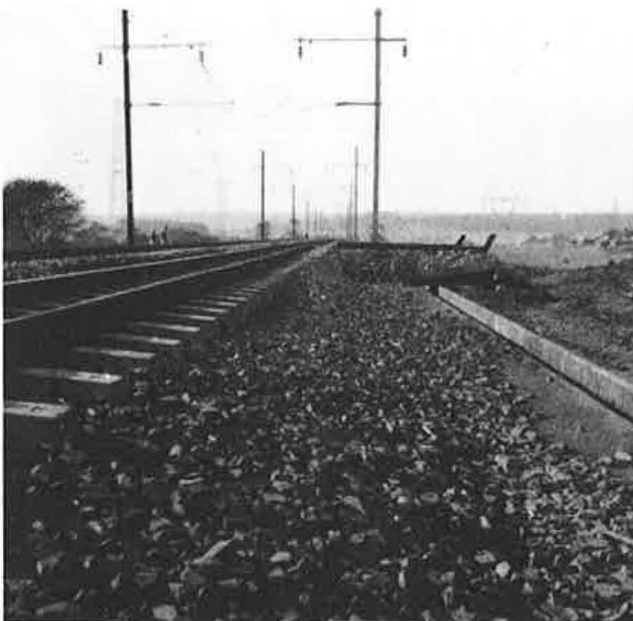
Fig. 2 Shifting of ballast
