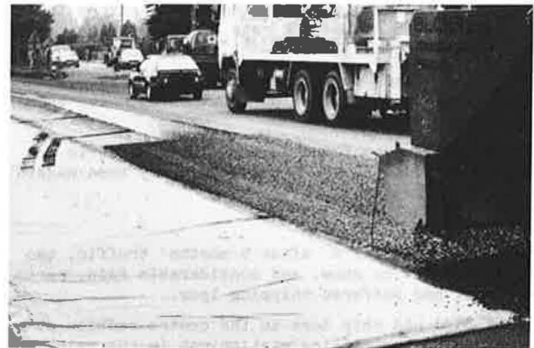
Trial Site 84/1 Overspray and Chipping
