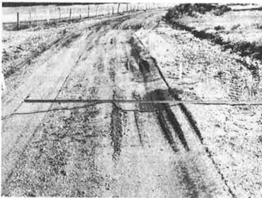
Fig. 11 : Ruts on the control section
