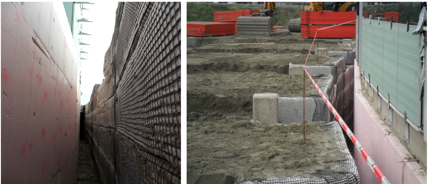
Figure 8. 14 m high earth pressure relief at an office building using GRE to leave a gap between earth embankment and wall
