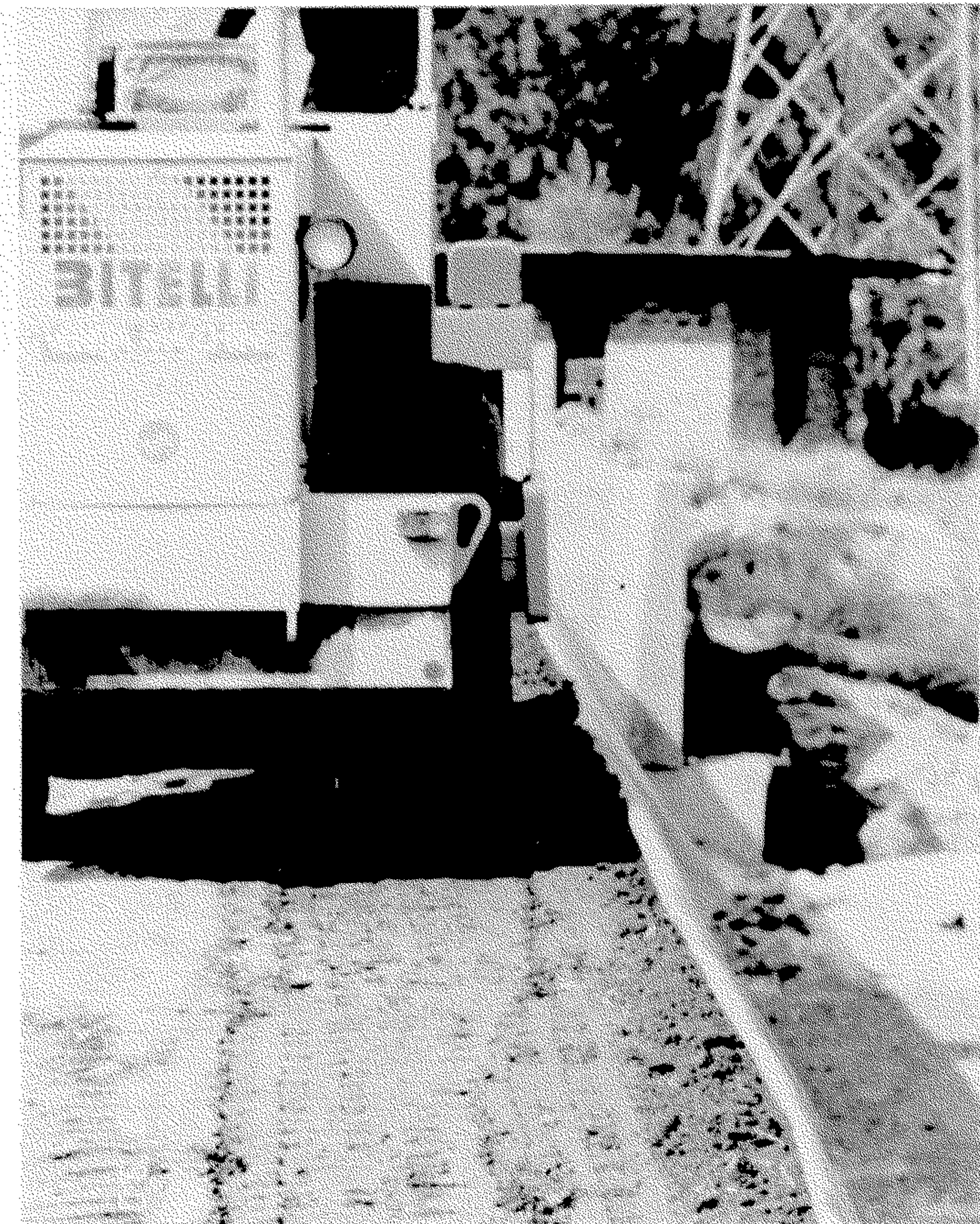
Fig. 5 4 t drum vibratory roller compacting the fill of a GRSS right to the face of the structure.
