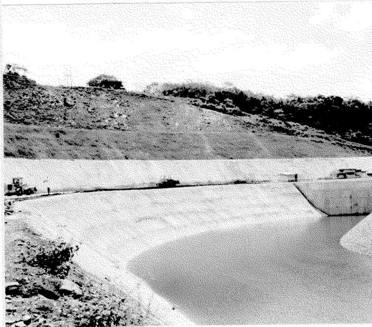
Figure 6 Completed retaining berm in the upper part of the left slope of the spillway approach channel.
