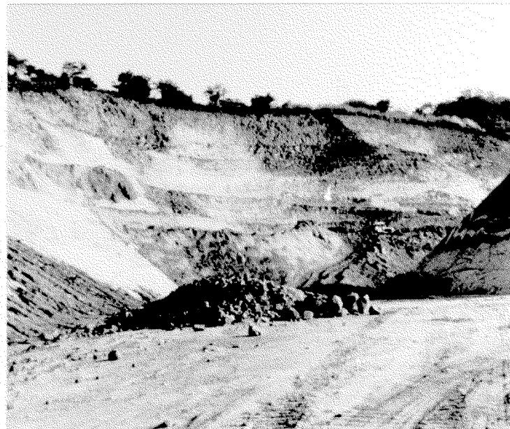
Figure 1 Sliding area of left slope of the spillway approach channel.
