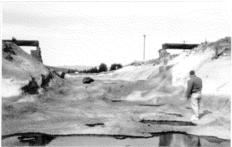
Figure 8 - North Unit Canal test sections 6 through 9. Completed canal section with 75-mm shotcrete lining.
