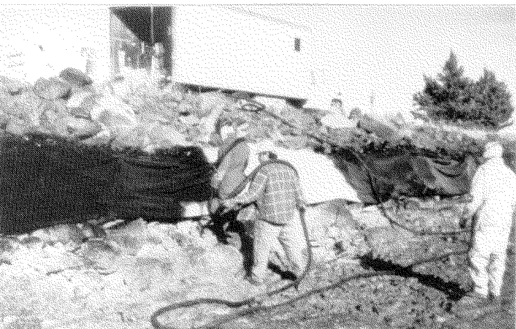
Figure 6 - North Unit Canal test sections 3 and 4. Application of protective coating to geotextile.
