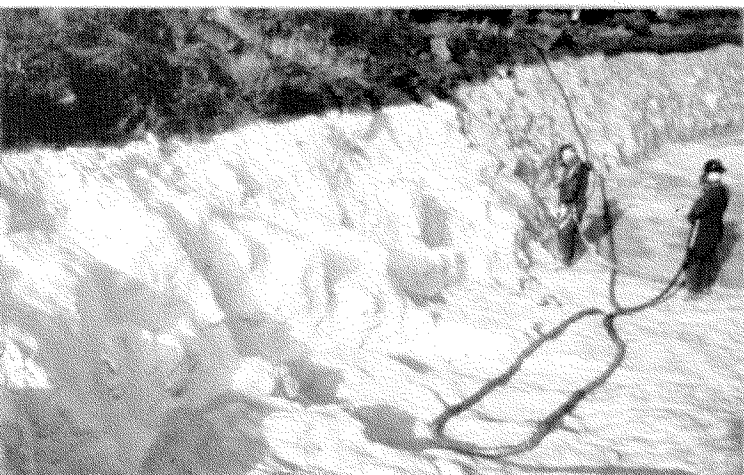
Figure 5 - North Unit Canal test sections 1 and 2. Spray application of polyurethane foam and coatings.
