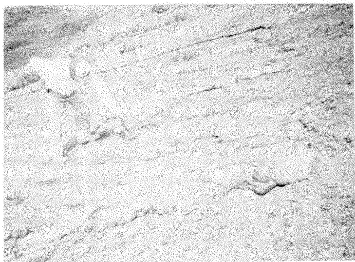
Fig. 1 Asphaltic revetment shrinkage at Zumpango Lagoon
