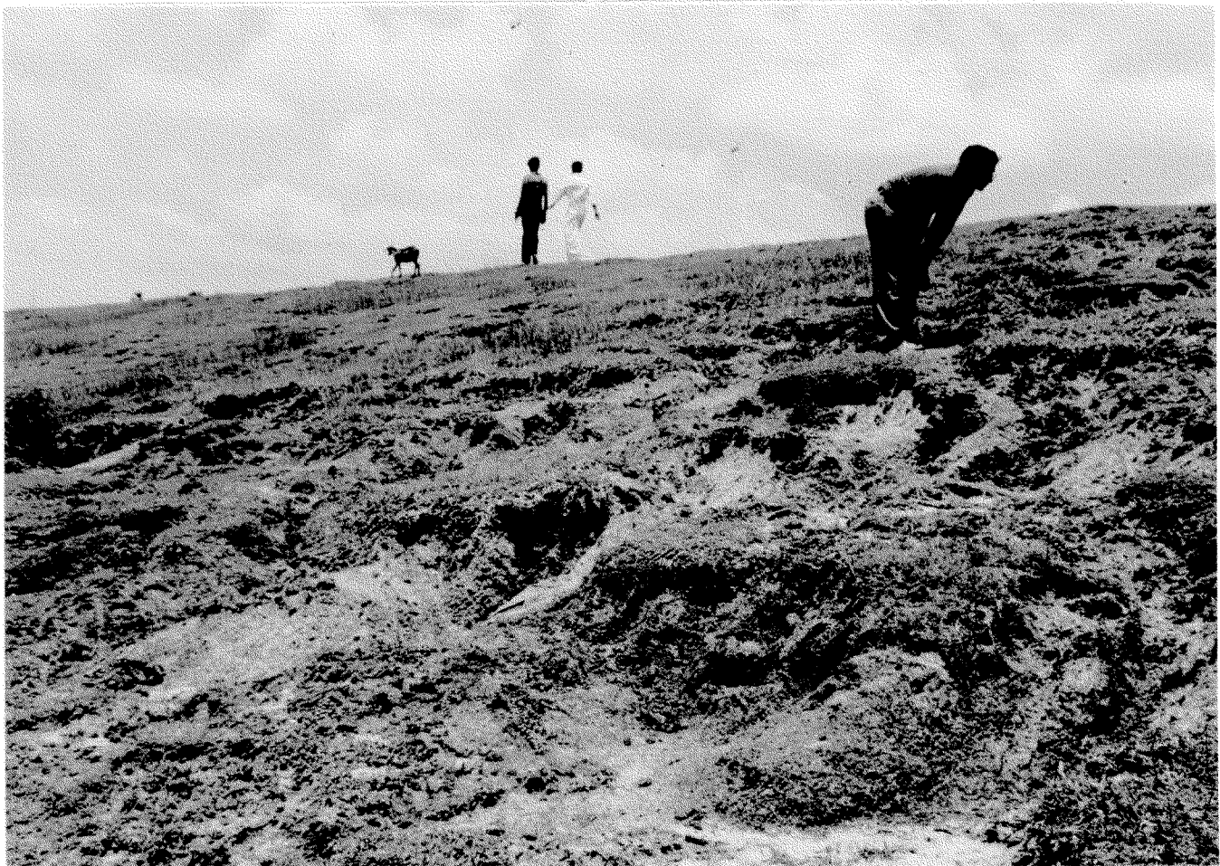
Fig 4. Embankment slope treated with geojute but with inadequate maintenance showing some distress to grass
