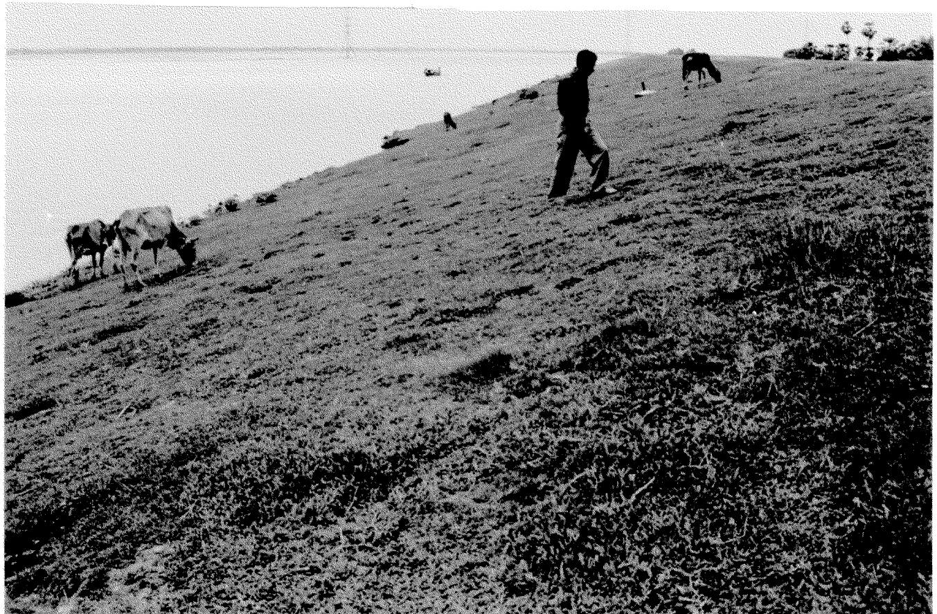
Fig 1. Embankment where Geojute was laid and grass blocks were fixed and maintained, showing controlled erosional vegetation
