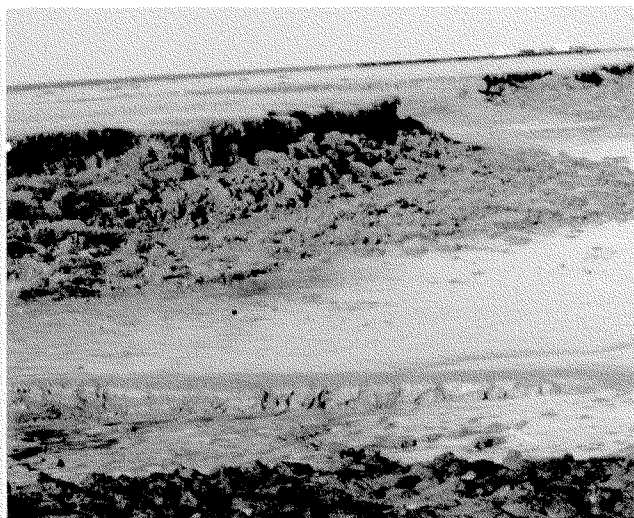
1. Erosion of river bank in Nayachor Island under Calcutta Port Trust, Haldia.
