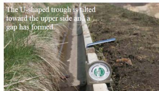
Fig. 2 Frost heaving damage to a berm on a cut slope
