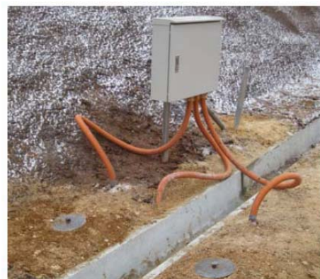
Fig.7 Instrument installation status
