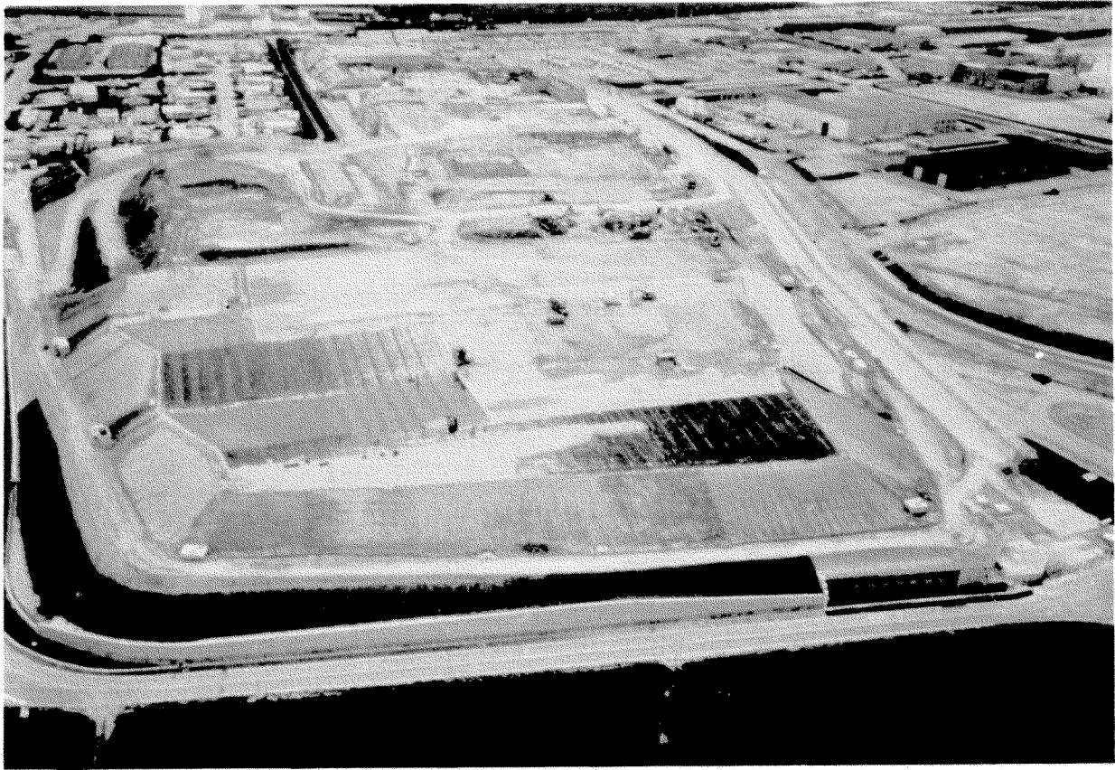
General view of the bituminous geomembrane capping on the radioactive waste landfill
