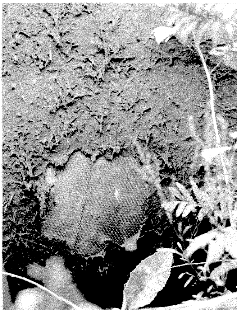
Fig. 9 Unprotected spot on the south side
