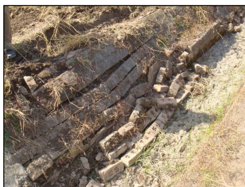
Photograph 3. Very high swelling and severe damage in Keshlu minor
