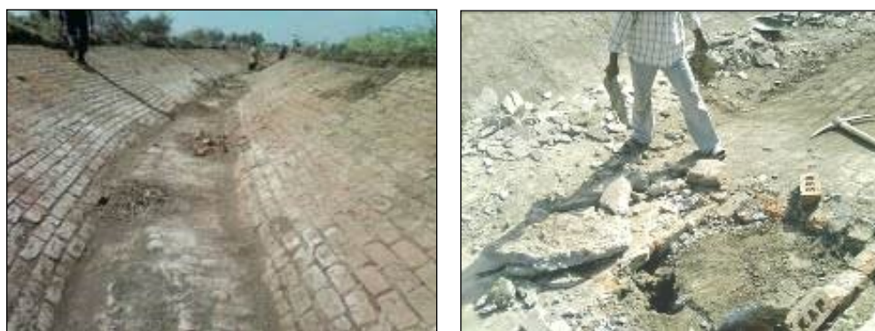
Photographs 1 and 2. Swelling of bed and sides and pipings from sides of Canal
