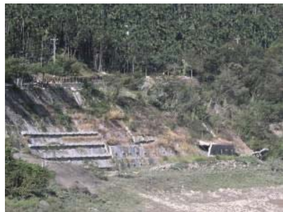
Fig. 1 Severely damage of original slope
