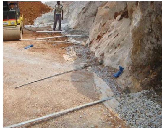
Fig. 5 A view of the steel strips provided at the interface of existing ghat road
