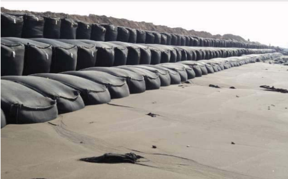
Fig. 8 Apron is covered by sediments in most length of the stretches
