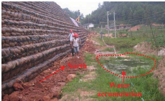
Fig. 4 Water accumulation at the slope toe.
