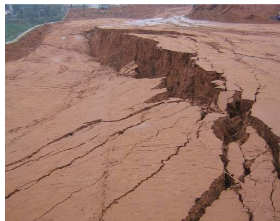
Fig. 11 Tension and pinnate fissures occurred at the berm of the slope.
