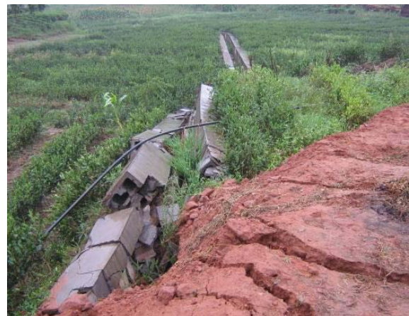
Fig. 10 Uplift and drainage ditch damage at the toe of the slope.
