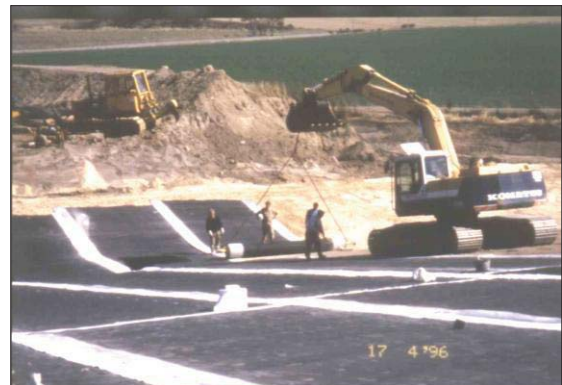
Fig. 2 Installation of the geosynthetic clay liner (GCL) as part of a geosynthetic cover system at the landfill Neu Wulmstorf near Hamburg, Germany, 1996/97
