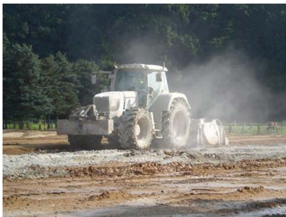
Fig. 7 Example of soil improvement by milling of binder (lime/cement) into the soil
