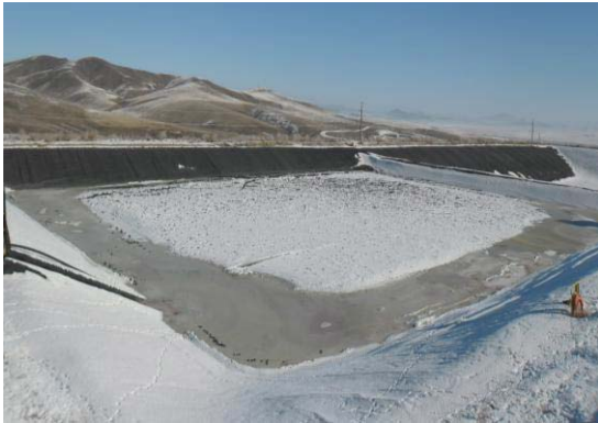
Fig. 6 HDPE lined chemical solution pond
