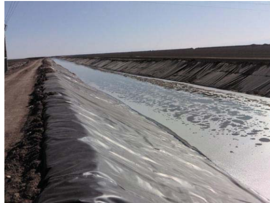
Fig. 5 HDPE lined channel transporting brine in Qinghai Province, China
