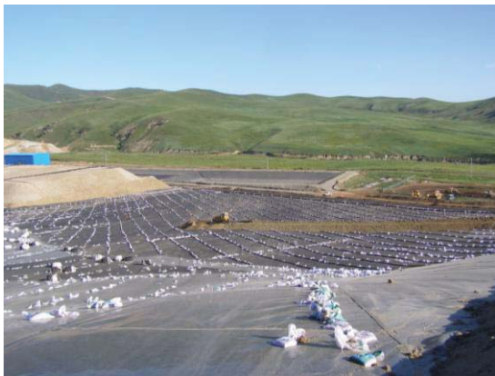
Fig. 7 Heap leach pad system was lined Polyethylene geomembrane at a mine site.
