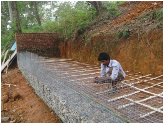
Fig. 7 Placing of gabion boxes and Laying of bamboo reapers for the second layer of retaining wall
