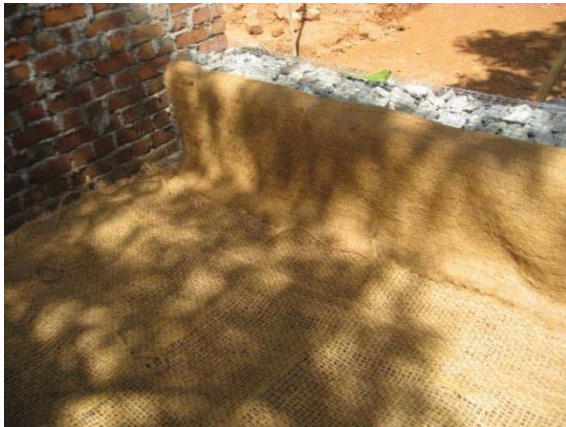
Fig. 8 Laying of woven coir geotextile as reinforcement and non-woven coir geotextile as filter
