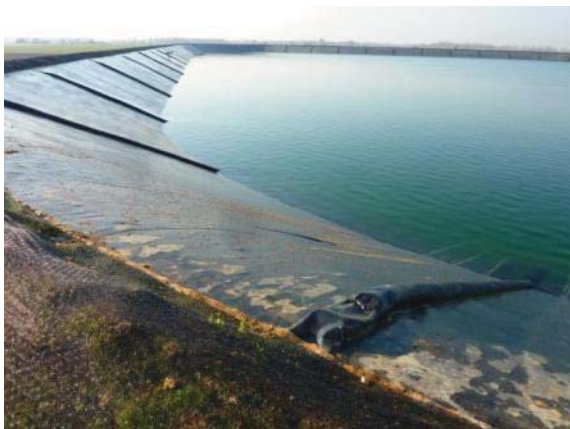
Fig. 37 Wind ballast with PE bags filled with gravel and anchored on the crest
