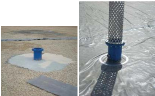
Fig. 24 Water outlet pipe at the bottom
