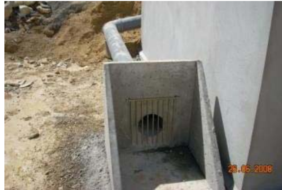
Fig. 26 Water drainage outlet
