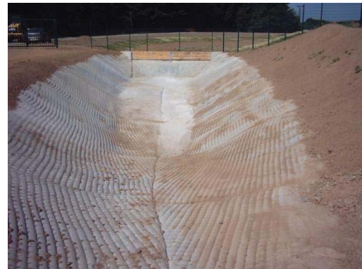
Fig. 14 Storm water basin with a geosynthetic concrete mattress as a sealing system.
