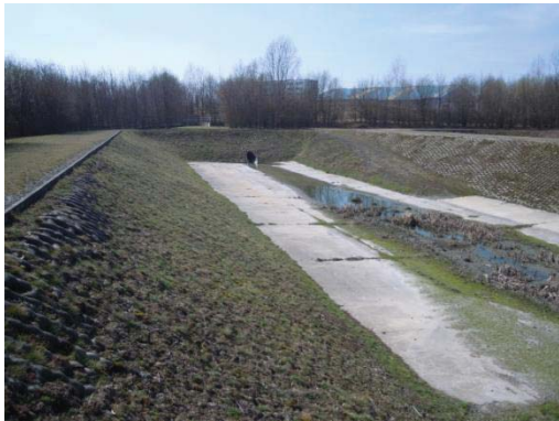
Fig. 16 Storm water basin: slopes covered with a geosynthetic concrete mattress (type Crib ) 19 years after installation.
