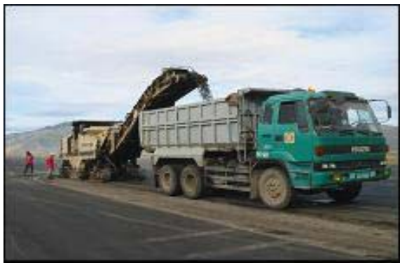
Fig. B1 Runway centerline milling and cleaning of existing pavement 50mm thick.
