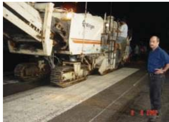
Fig. A1 Milling of the center line 100mm into the existing old asphalt concrete
