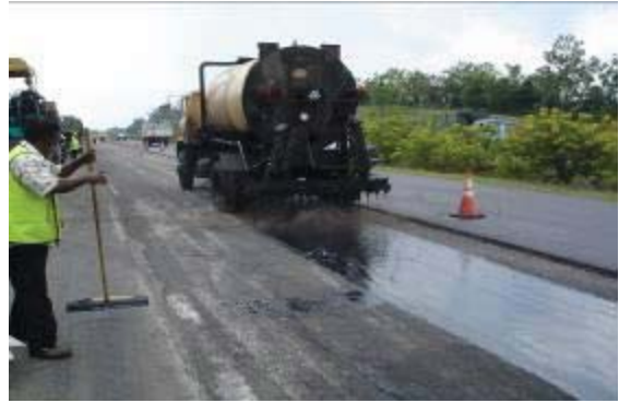
Fig. D2 Polymer modified bitumen tack coat was applied to the old pavement.paving rig.
