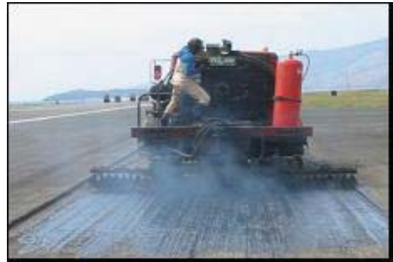
Fig. B2 Initial run of tanker controlled spray bar with 1.1kg/m 2 rate of application.
