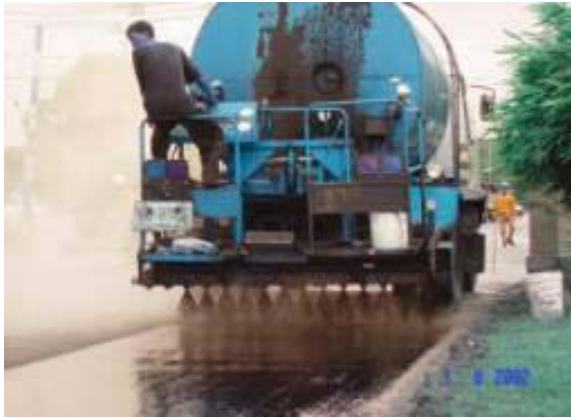
Fig. A3 Spreading of pure bitumen tack coat using metered dozing system.
