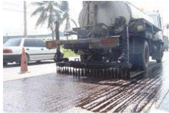
Fig. E2 Spraying of Cationic Rapid Setting (CRS-2) bitumen emulsion tack coat.
