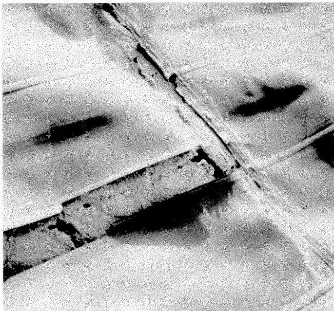
Fig. 21 Crack in an HDPE geomembrane located partly along a seam and partly along an area of greater thickness resulting from the manufacturing process.
