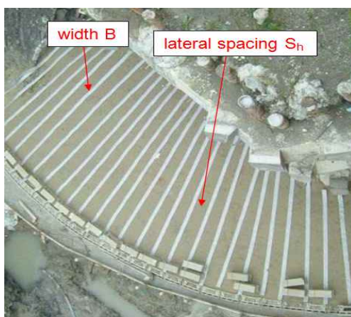
Fig. 5. Internal drainage system made up of geocomposite strips
