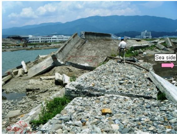
Figure 3. Destroyed seawall at Takata-matsubara (Kuвано et al., 2012, 2014).
