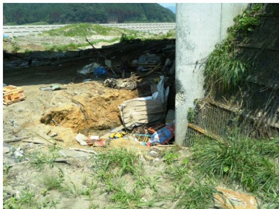
Figure 11 Scouring at the abutment of the Nanakiri overpass (Kuwano et al., 2012, 2014).
