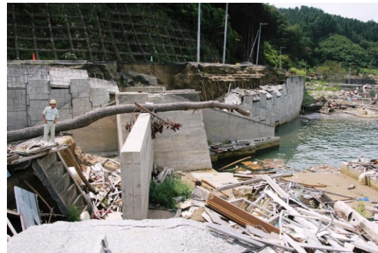
Figure 6. Close-up view of damaged RSW1 (Kuвано et al., 2012, 2014).
