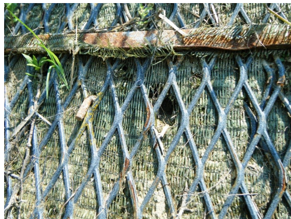
Figure 12 Slight damage at the expanded metal mesh facing of RSW3 (Kuwano et al., 2014).
