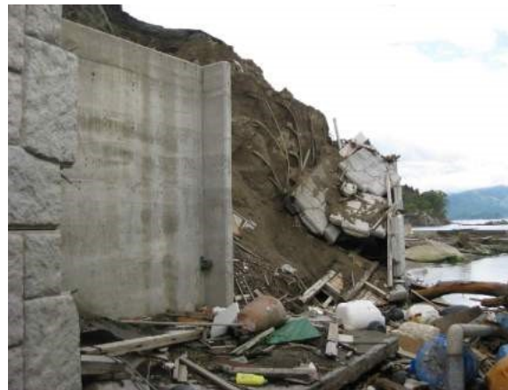
Figure 8 Erosion of the backfill of damaged RSW1 (courtesy of Dr. Otani, Hirose Corp.) (Kuвано et al., 2012, 2014).
