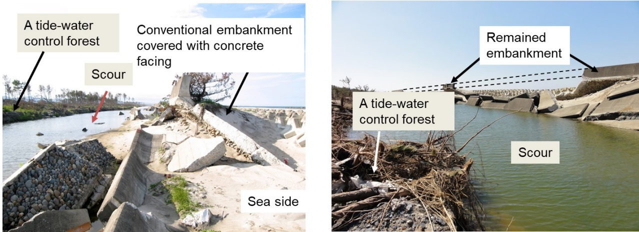
Figure 31. Damage of coastal dike and its surroundings.
