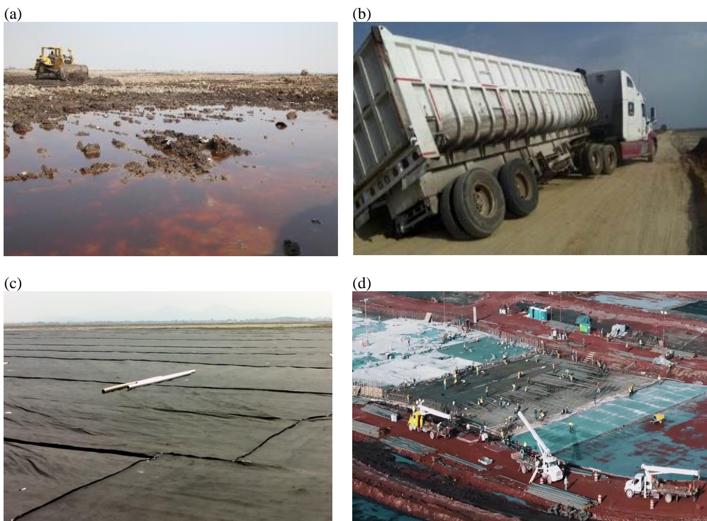
Fig.8. Case study involving subgrade stabilization: (a) View of the saturated clay at the New International Airport of Mexico City before construction; (b) Evidence of significant problems with low bearing capacity; (c) Placement of geotextile to create a working platform; (d) construction operations
