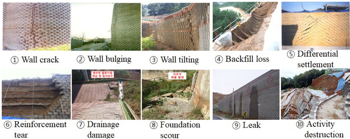
Figure 1. Damage type of reinforced earth retaining wall(Some of these figures use press releases)
