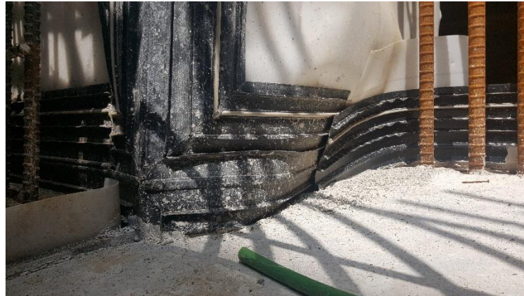
Figure 1. Poorly installed waterstop in tunnel construction
