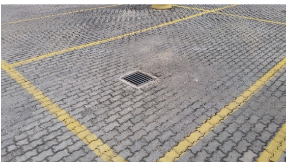
Figure 7. Detail of the surface drainage, by means of box with grid, interconnected to the drainage system with drainage geocomposite .
