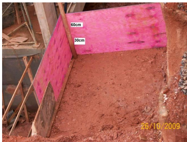
Figure 20. A wooden structure, mounted on a retaining wall, to contain a soil load (overload).
