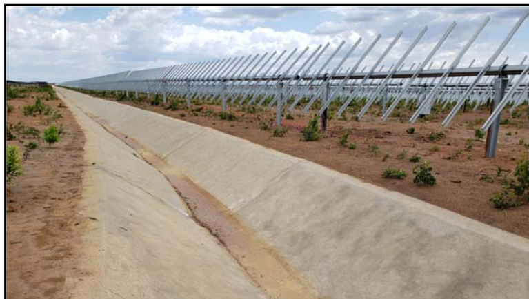
Figure 12. Photovoltaic plant in São Gonçalo do Gurguéia, PI
