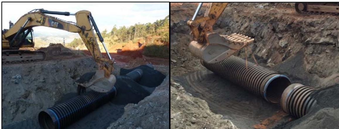
Figure 9. Installation of pipe sections without manual assistance as required by mine safety.
