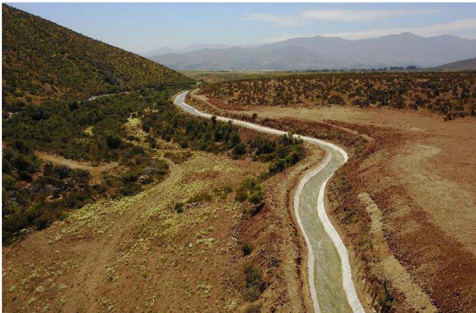
Figure 1. Aerial view of a completed section of phase two installation at Bellavista canal
